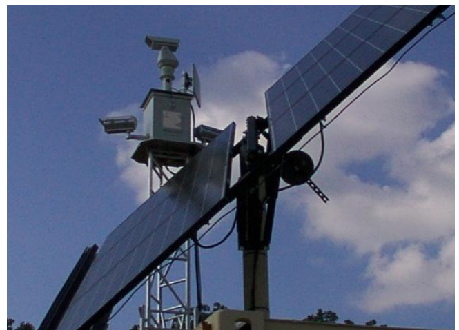
Solar Powered Surveillance System - Fort Leonard Wood Missouri
